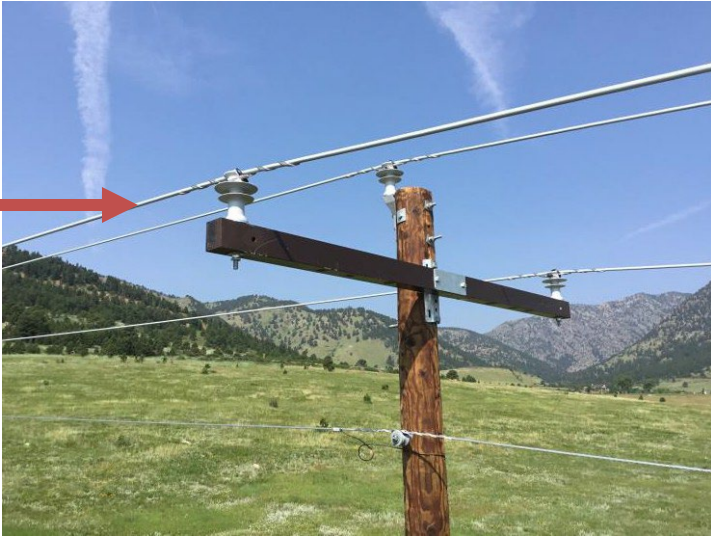
Three-phase covered conductor. (Blue Mountain 2)
