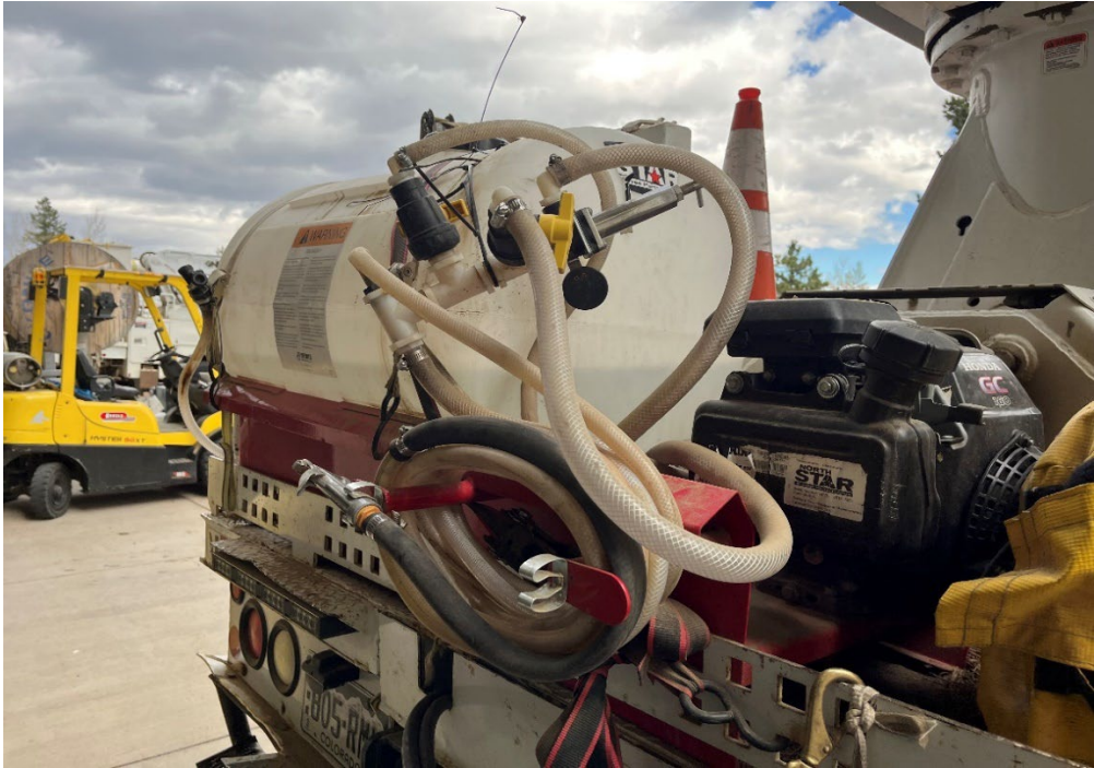
Water tanks on digger derricks for dust control and spot fire control.
