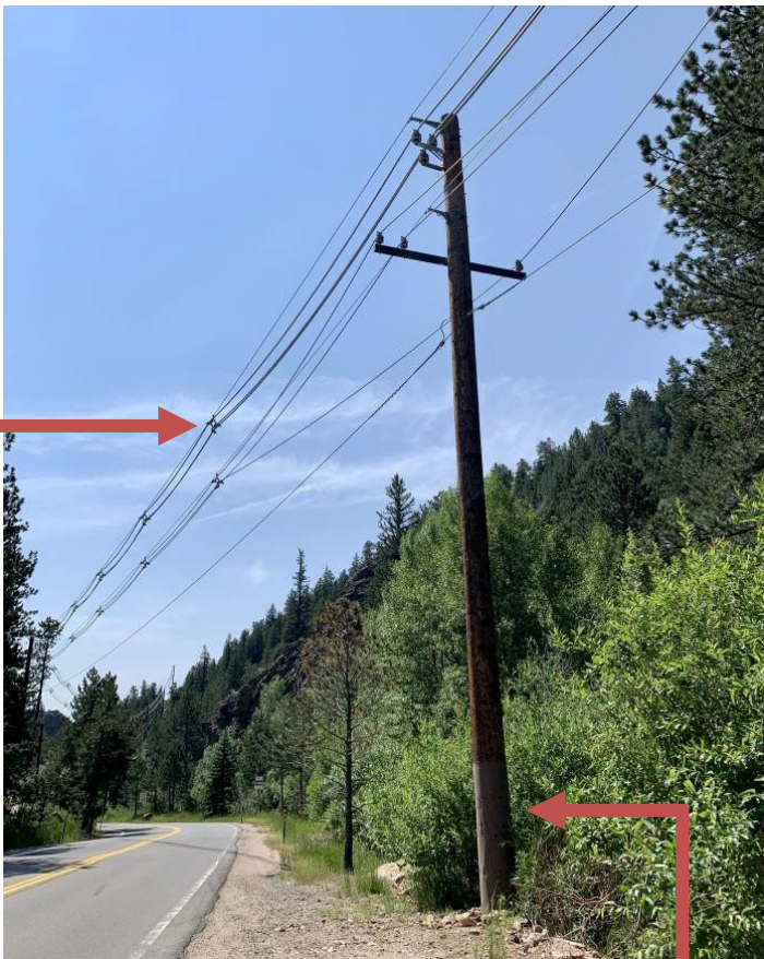
Hendrix spacer cable. (Sub-transmission – Plainview 1) (Distribution – Under build Crescent 7)
