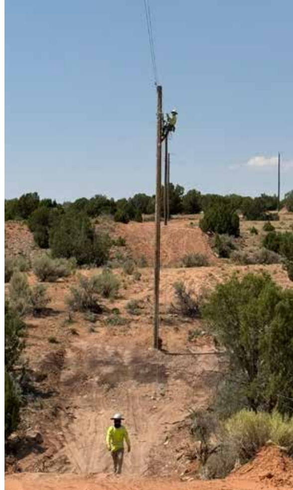
Line crews work to set poles and hang line in the New Mexico region of the Navajo Nation. Loose dirt and rocks along with scorching heat made conditions challenging.
